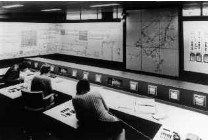
This photo, taken around 1970, shows the control room of Gasunie in Groningen, where the central distribution of Dutch natural gas was coordinated. The control panel shows the network of pipelines across the Netherlands.
